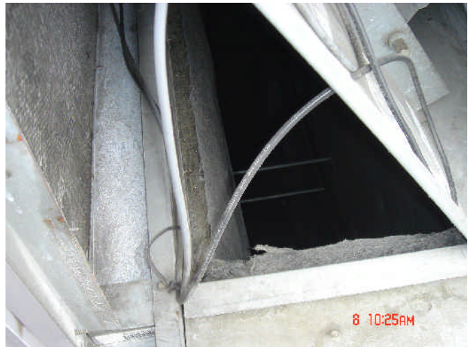
Close up of dirty plenum and unit boards. [FE] [CR]
