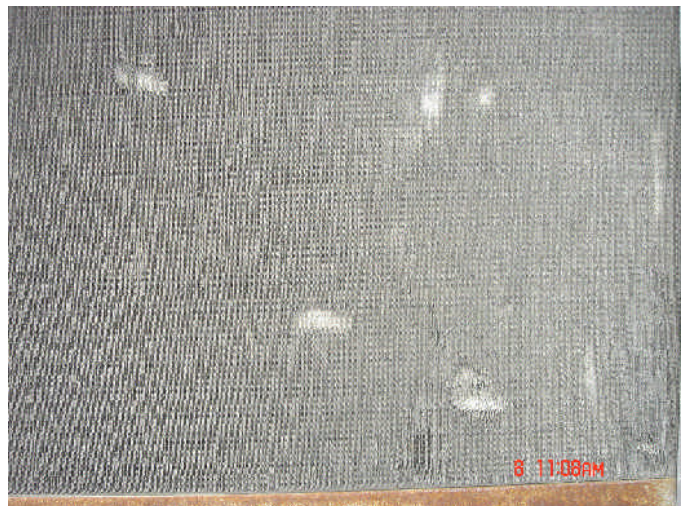
More damage to the exterior condenser coil fins. [FE] [CR]
