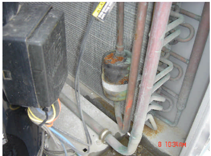
Close up of the rusted refrigeration dryer. [FE] [CR]
