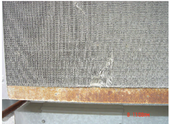
Damage to the exterior condenser coil fins. [FE] [CR]
