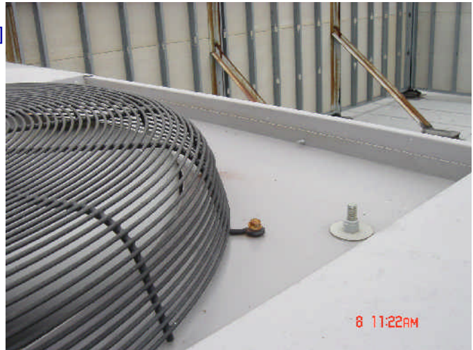
Condenser air discharge fan with loose mounting screw. [CR]
